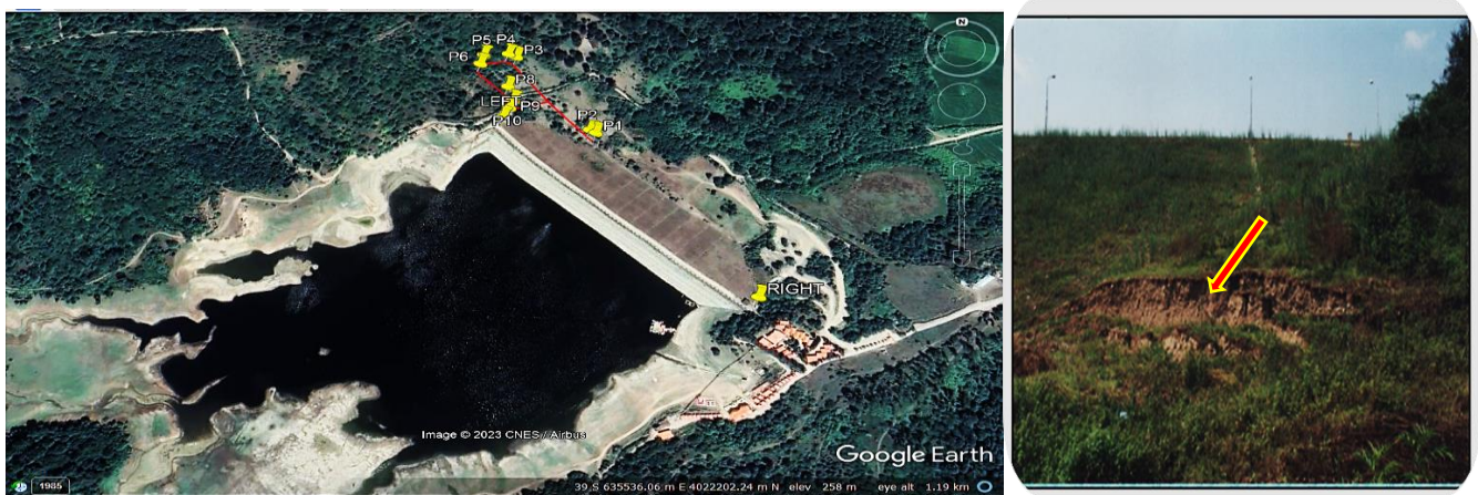
Fig. 4: Landslide downstream of the left abutment and shallow sliding at the dam toe
