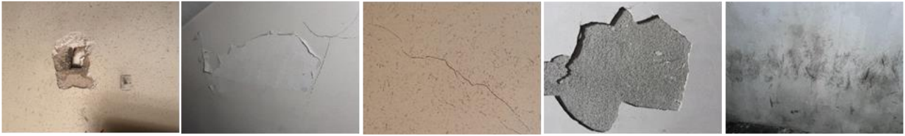
Fig. 2: Examples of some defects during inspection
