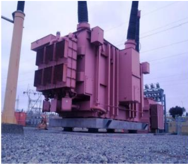
Fig. 7: Seismically isolated transformer in Vancouver
