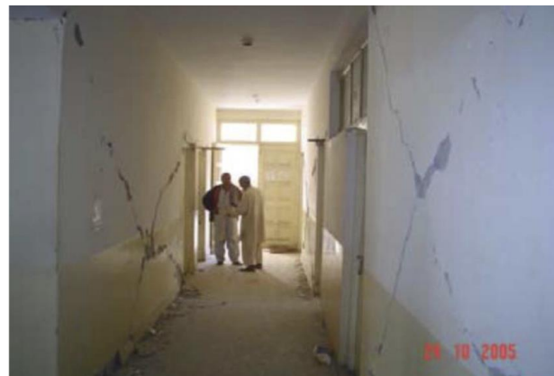
Damages in Brick Masonry Buildings in 2005 Kashmir Earthquake
