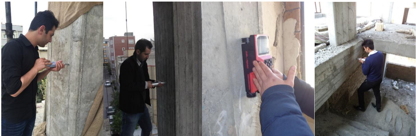
Fig. 1: Sample pictures of non-destructive tests by the engineers of Mandegar Structures Q.C. & Inspection Company
