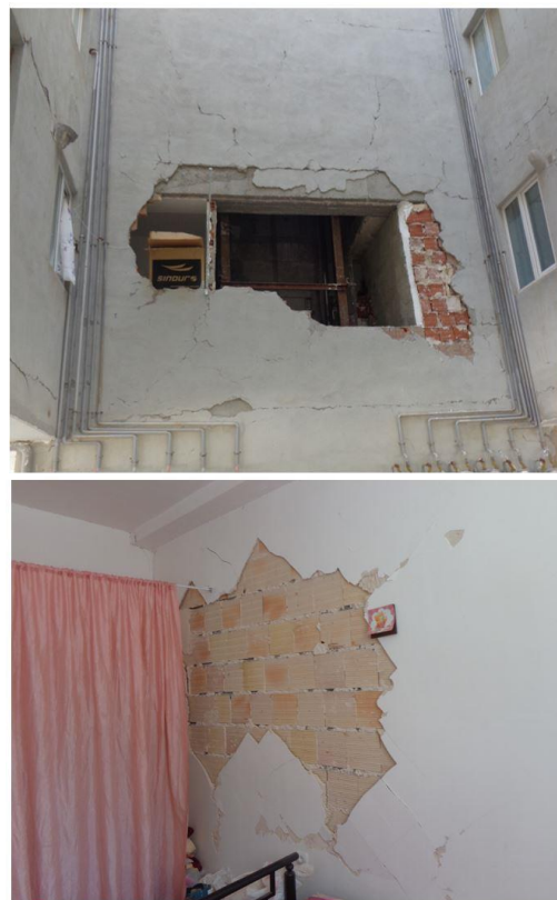
Fig. 1: Non-structural members damage in the Bojnord 2017 earthquake. The pictures were taken by the engineers of the Mandegar Structures Q.C. & Inspection Company.
